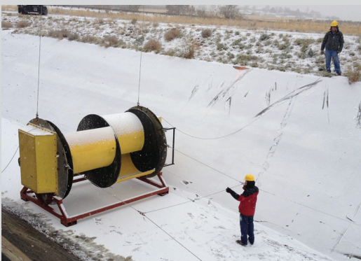
Dry install test run of the C-3 turbine in the Federal Bureau of Reclamation's Roza Canal
